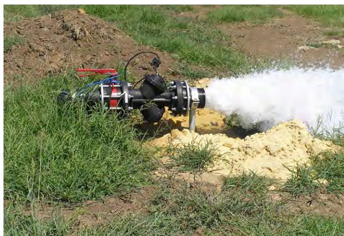
Using piped head ditches instead of open-channel ditches can result in a 12 to 15 percent saving on-farm.
