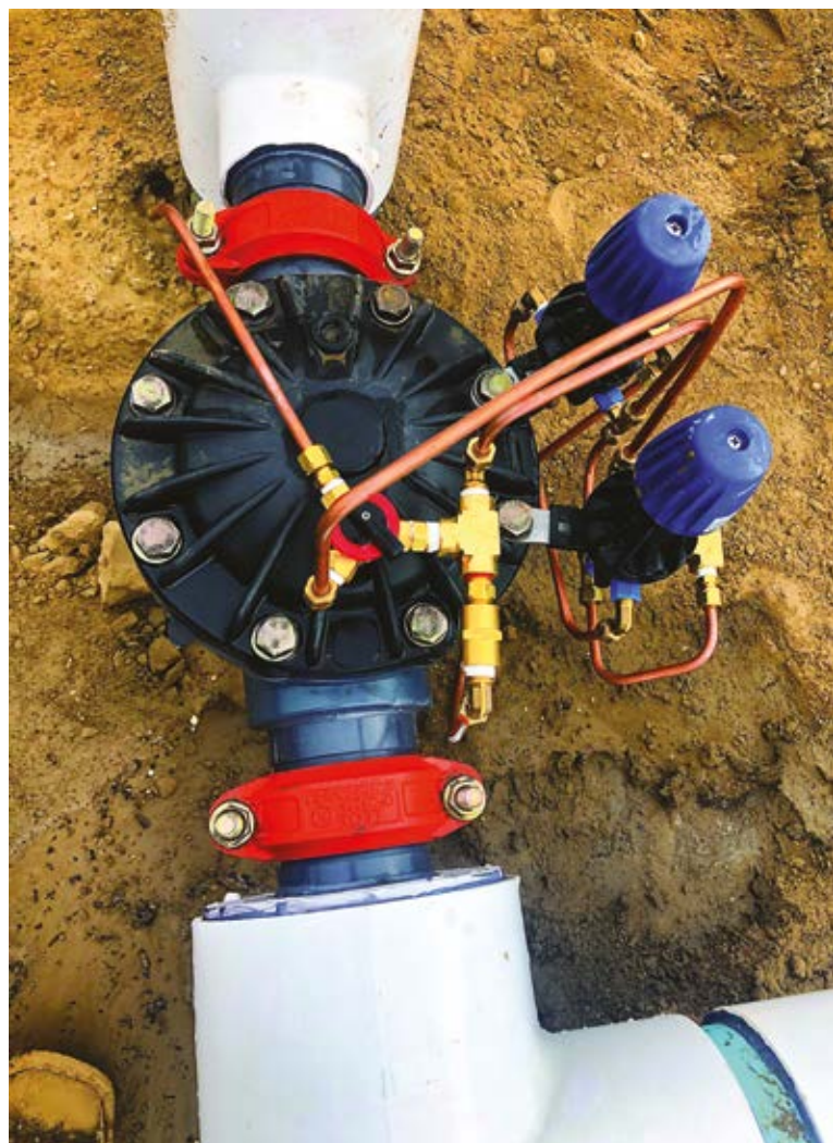
This pressure reducing and sustaining valve has a three-way manual selector and can sustain upstream pressure and reduce downstream pressure.
