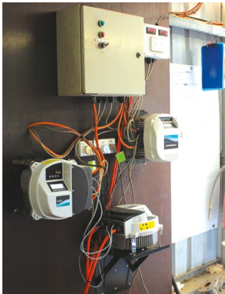
Three controllers are installed in the pump shed to control three multi-stage pumps which supply irrigation water from a water storage to the Donnybrook nursery site.
